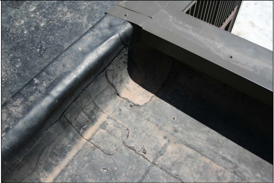
Notes: Glued patches and seams at southwest corner.
