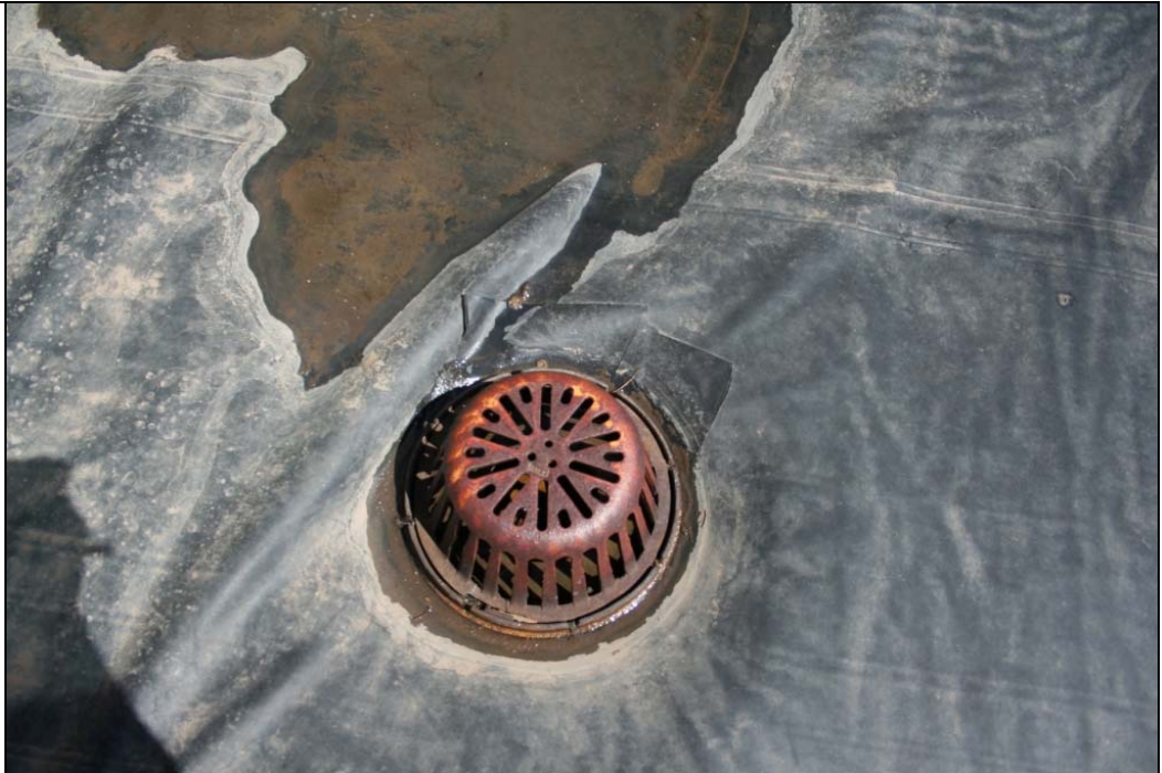
Notes: Patches south of roof drain.
