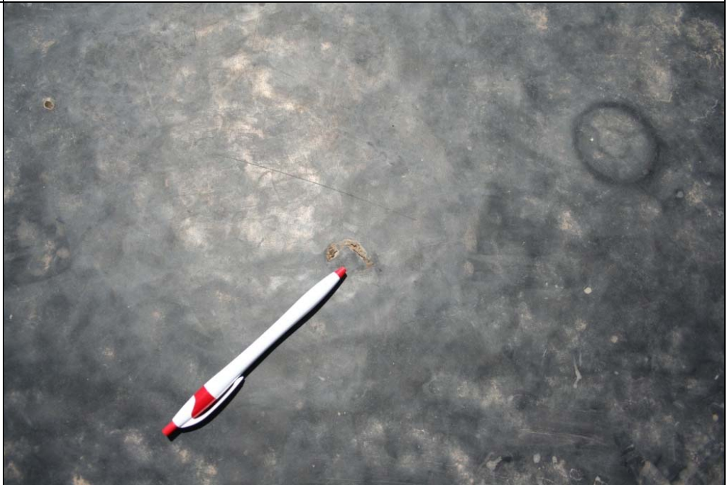
Notes: Detail of Photo 5. Hole appears to have been previously fixed.
