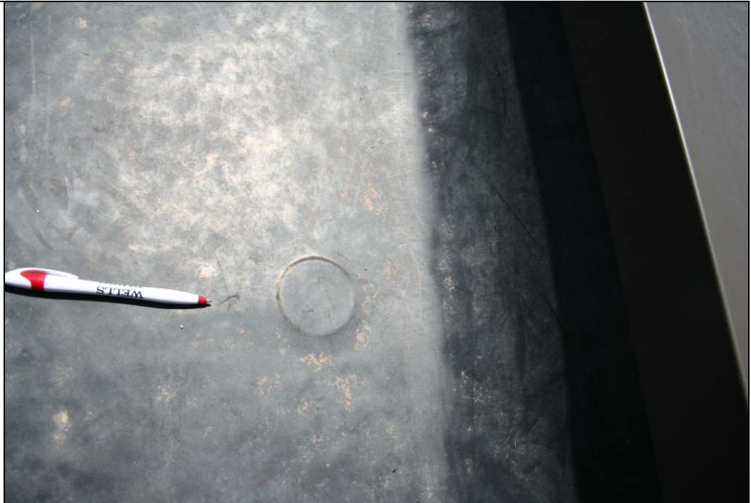
Notes: Hole in membrane, northwest corner.
