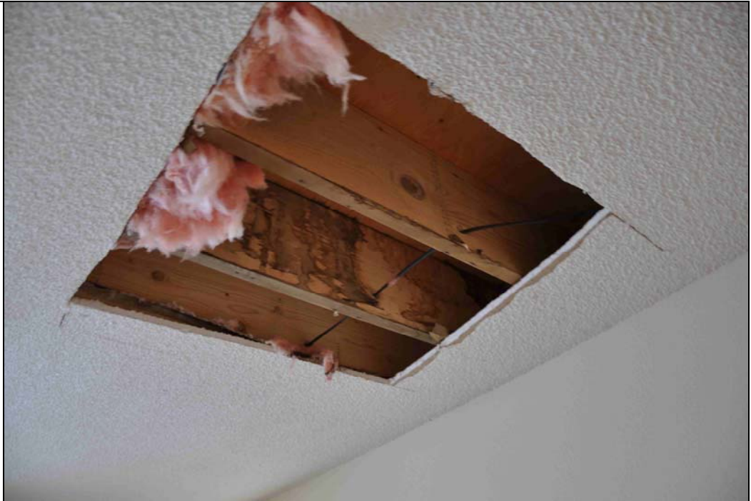
Notes: CBL Interior photo of drywall damage. Damaged area has been removed.
