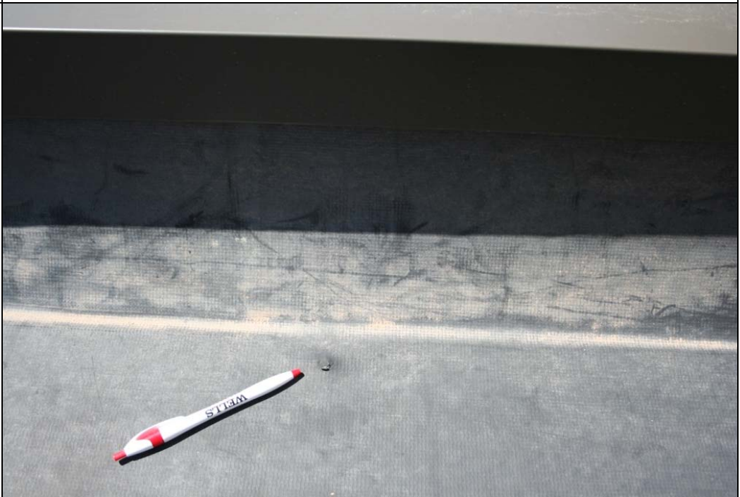
Notes: Detail of nail head protruding near overflow scupper.
