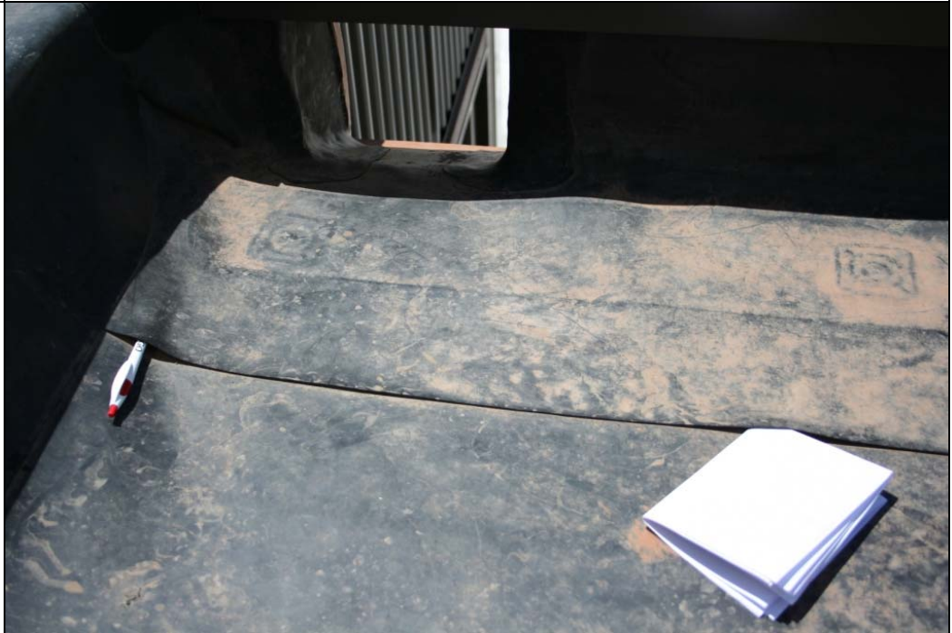
Notes: Seams not fully adhered at overflow scupper.
