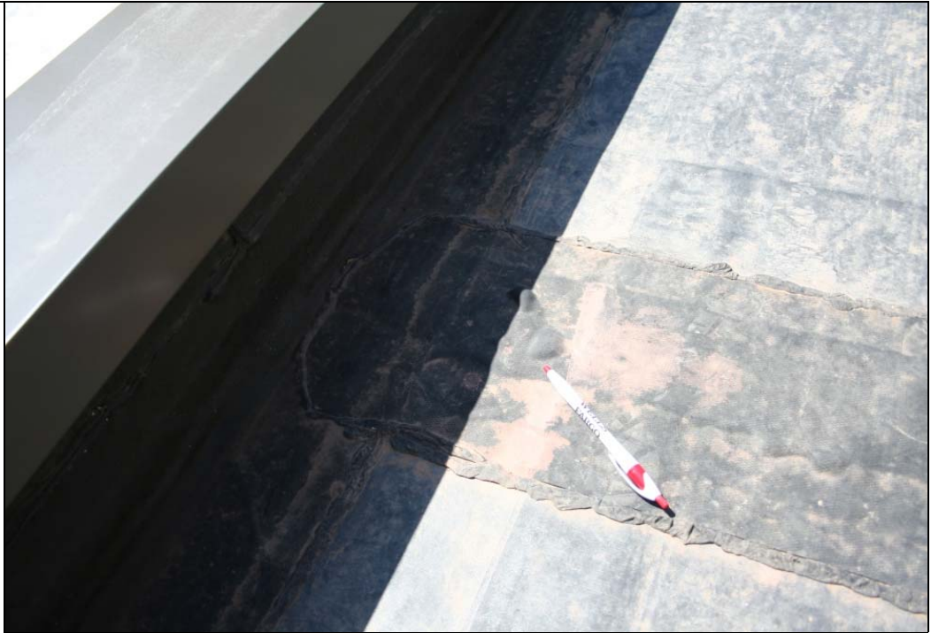
Notes: Bubbling in seam in multiple locations.
