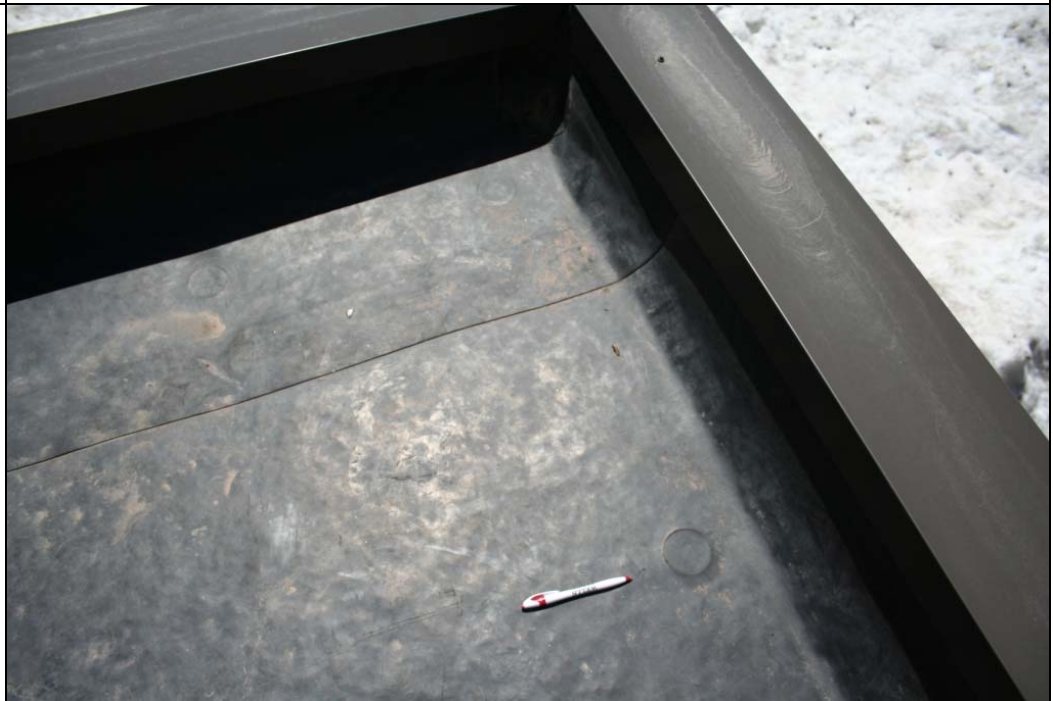
Notes: Location photo of hole in Photo 6.
