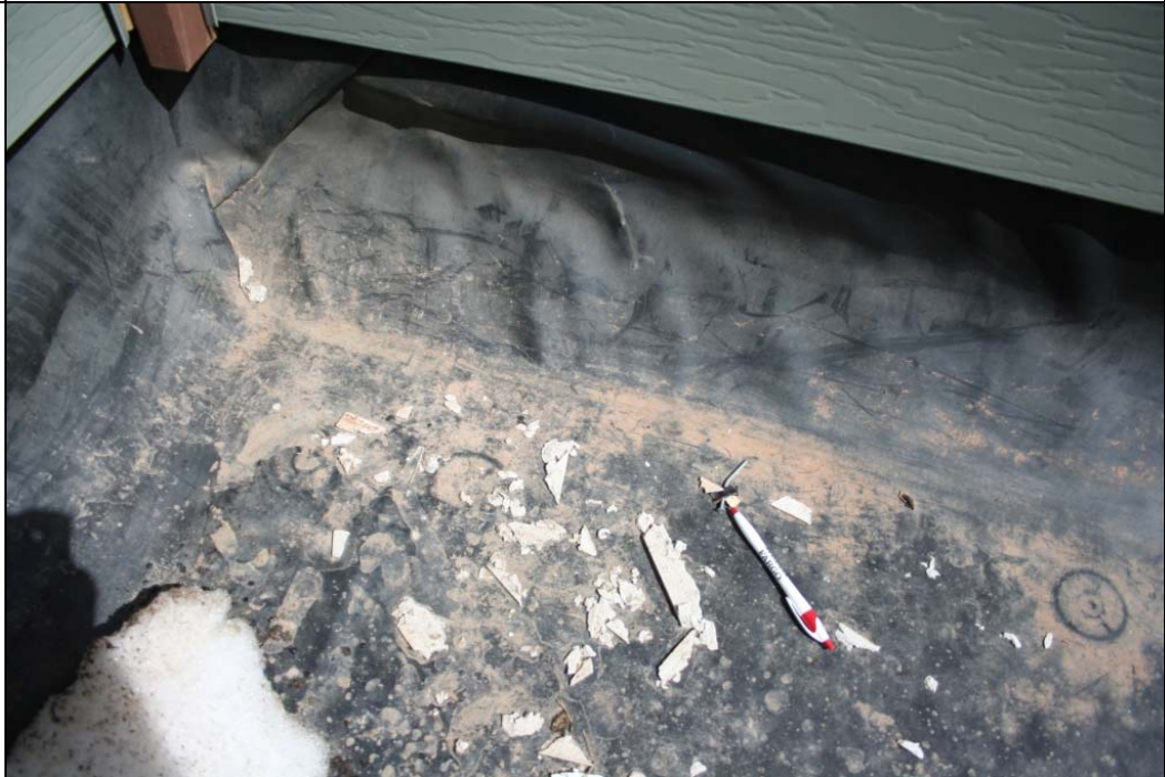
Notes: Construction debris and nail located in southeast corner. Nail removed.
