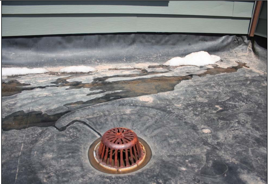
Notes: Membrane is not adhered to substrate.
