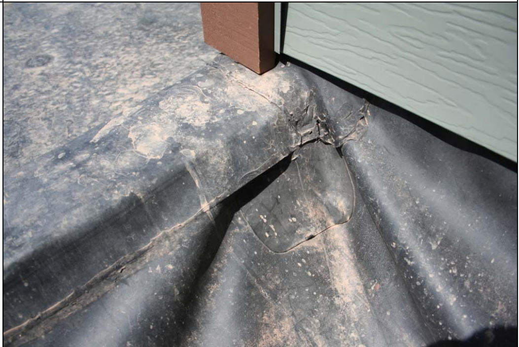
Notes: Large gap in lapped membrane on north parapet cap. Not necessarily indicative of leak.
