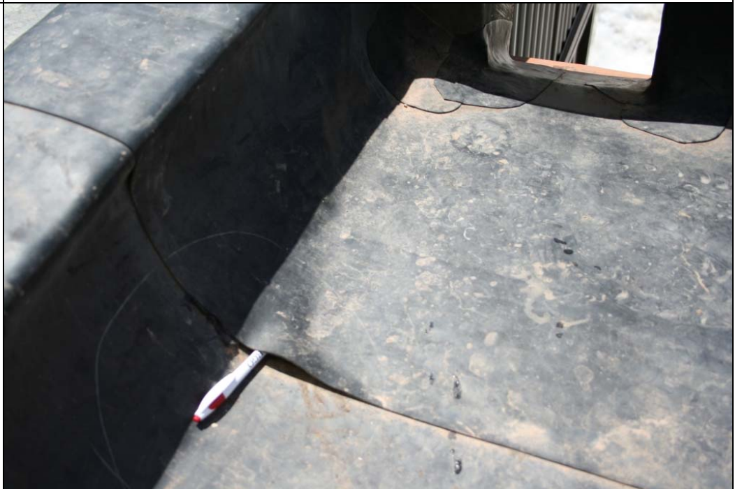
Notes: Seam not fully adhered at overflow scupper.
