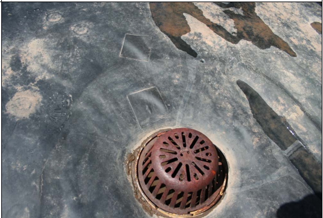
Notes: Two additional patches just north of the roof drain.
