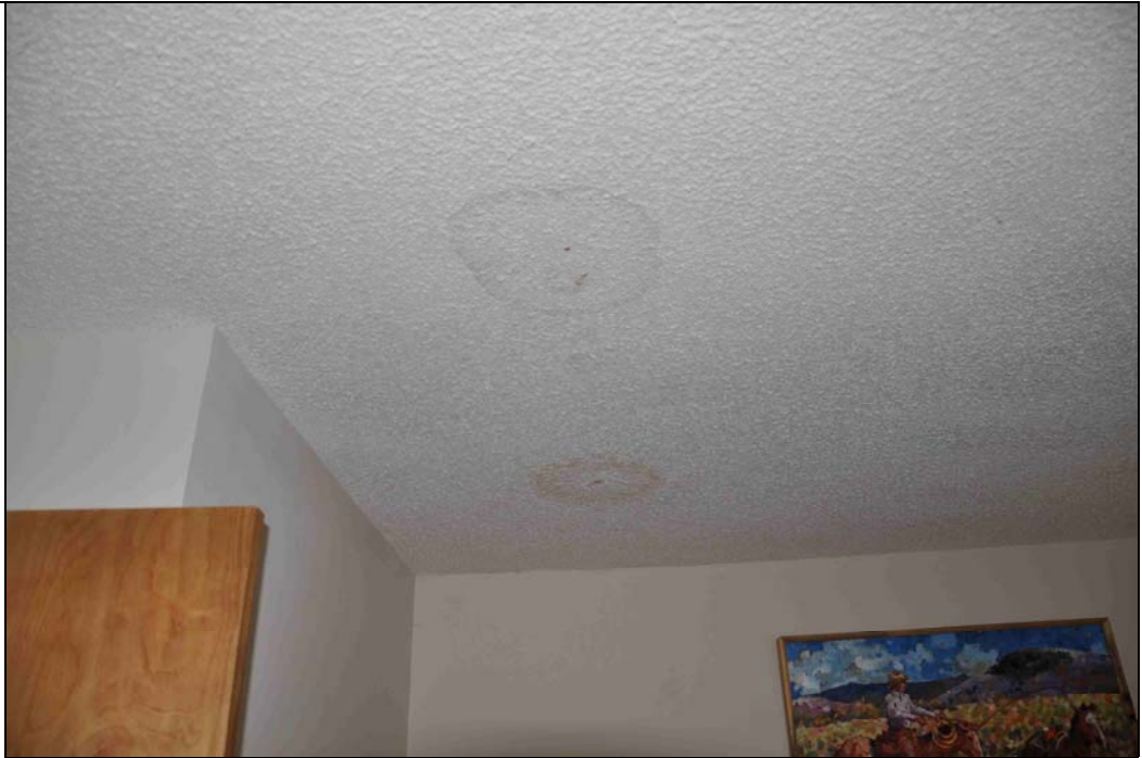
Notes: CBL Interior Photo of drywall damage.
