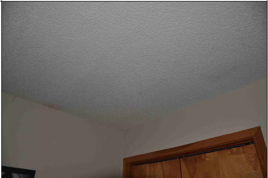
Notes: CBL Interior photo showing drywall damage.
