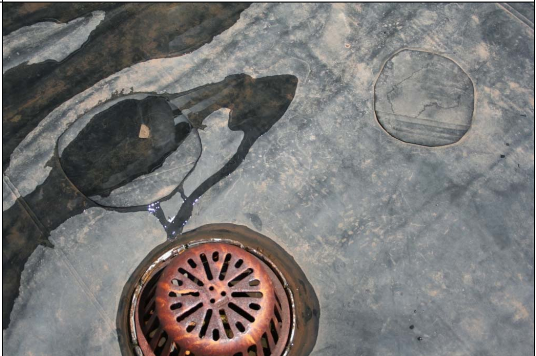
Notes: Detail of large patches south and southeast of drain.
