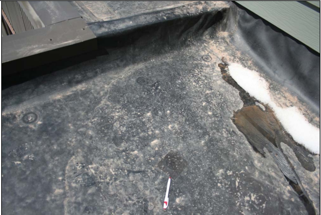
Notes: Existing patch in northeast corner.
