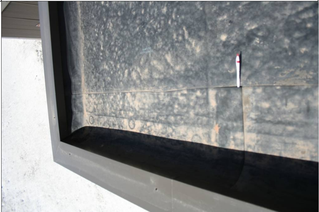
Notes: West seam not fully adhered.
