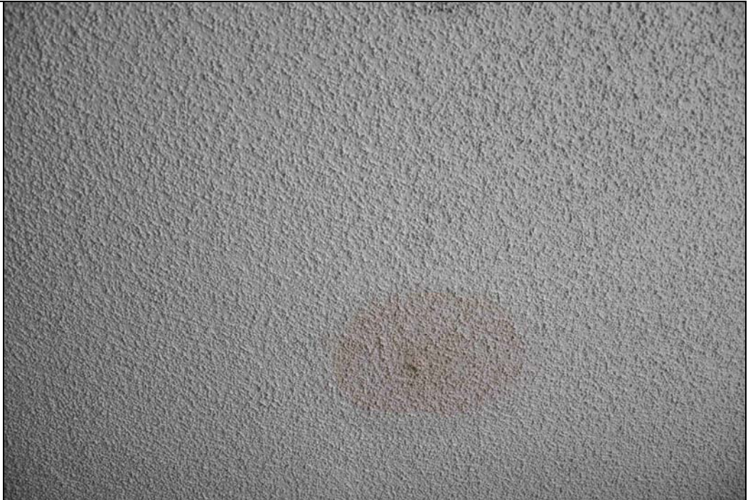
Notes: CBL Interior photo of drywall damage.
