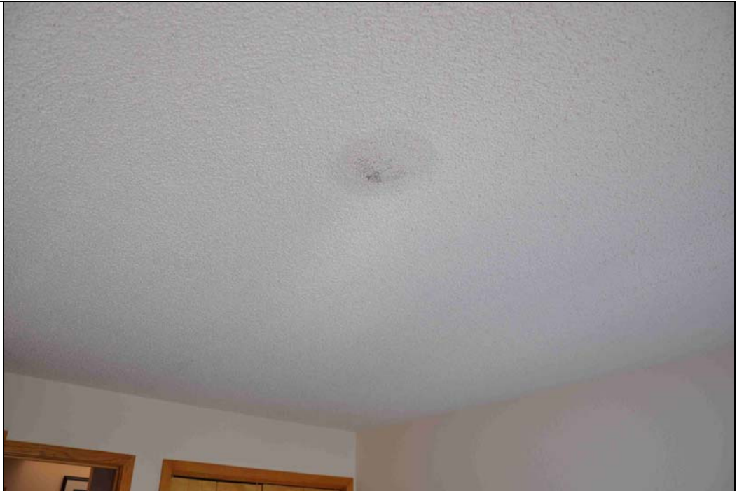
Notes: CBL Interior photo of drywall damage.
