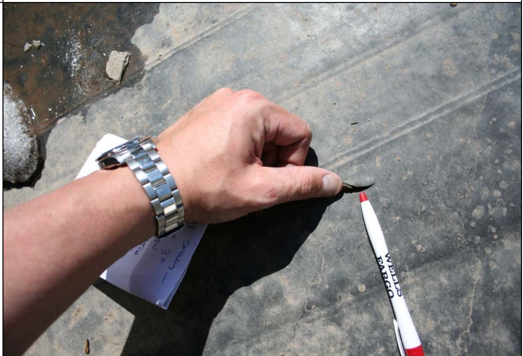
Notes: Detail of gash in Photo 5. Measures approximately 1" long.
