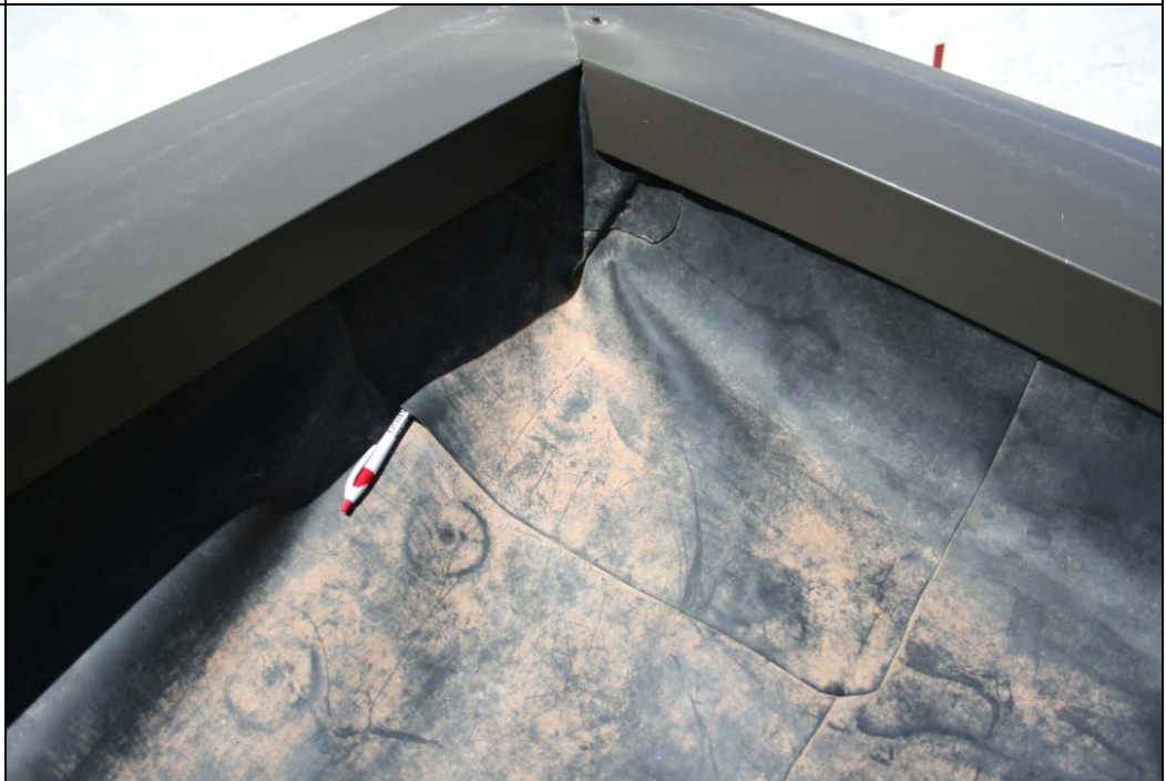
Notes: Seams not fully adhered at northwest corner.
