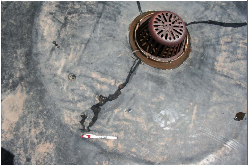
Notes: Location photo of holes and gash from previous photos. Pen marks location of gash. Note saturated substrate discharges water.
