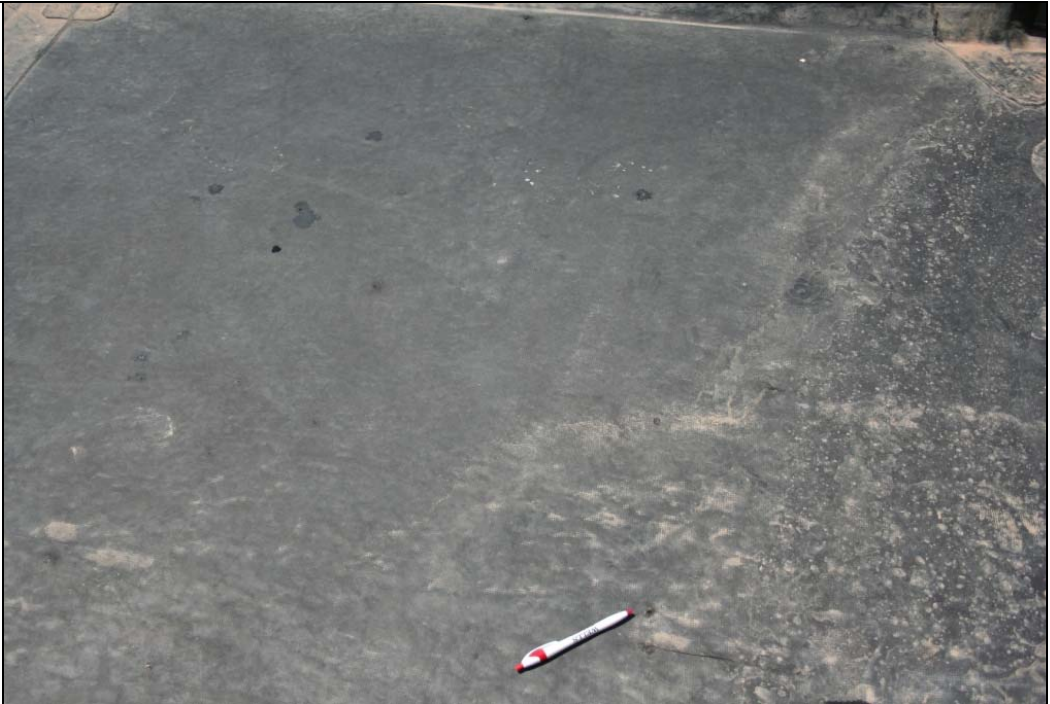
Notes: Nail heads protruding through membrane.
