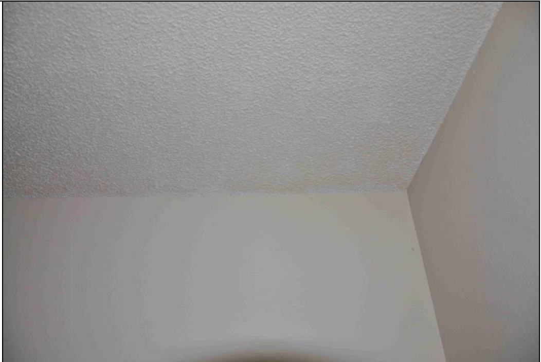
Notes: CBL Interior photo showing drywall damage.
