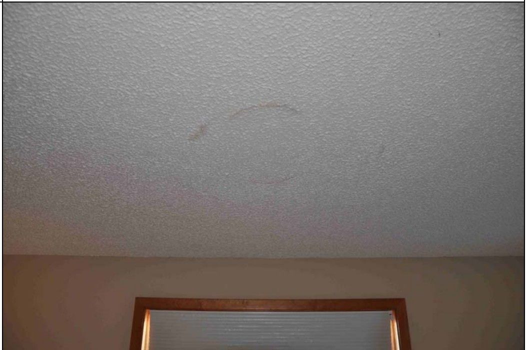
Notes: CBL Interior Photo of drywall damage.
