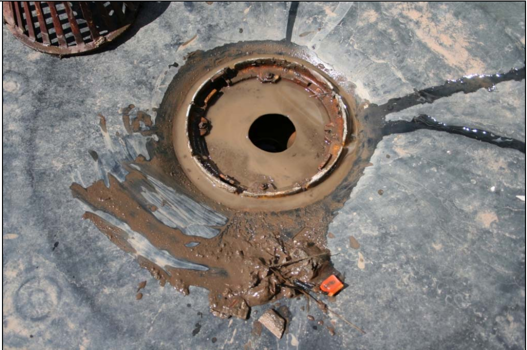
Notes: Debris removed from ring of roof drain.
