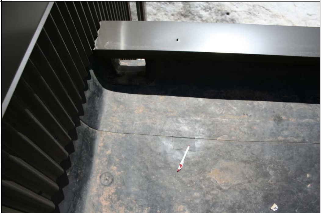
Notes: Patch located in southwest corner.
