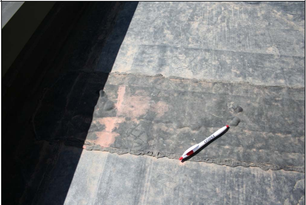
Notes: Bubbling in seam in multiple locations.
