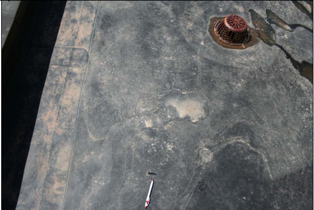
Notes: Hole in membrane approximately 4' southwest of roof drain.
