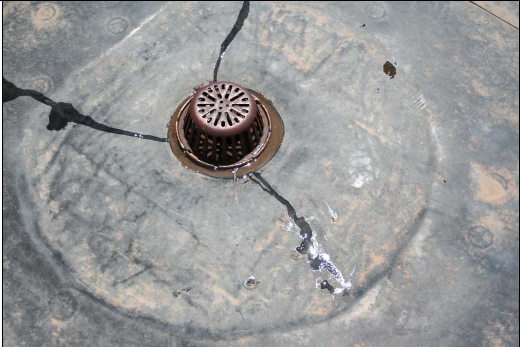
Notes: Location photo of holes and gash from previous photos.
