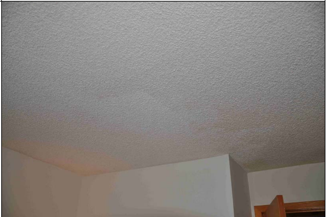
Notes: CBL Photo of interior drywall damage.
