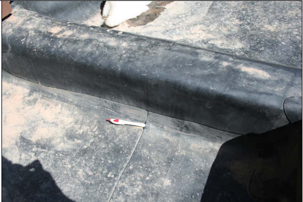
Notes: Seam at north side of parapet cap not fully adhered.
