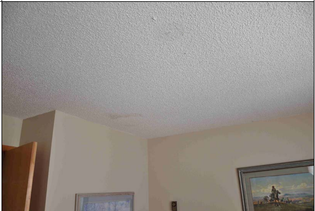
Notes: CBL Interior Photo of drywall damage.
