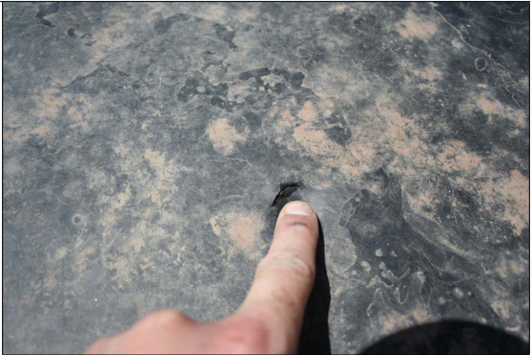
Notes: Detail of hole in membrane.
