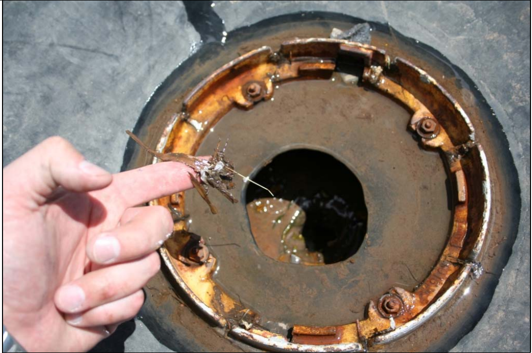
Notes: Debris in roof drain. Roof drain diameter is approximately 1-1/2".
