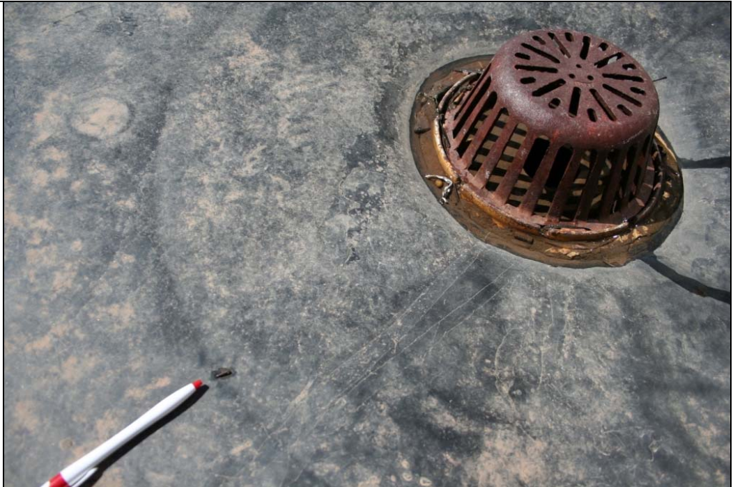
Notes: Staple has penetrated membrane southwest of roof drain.
