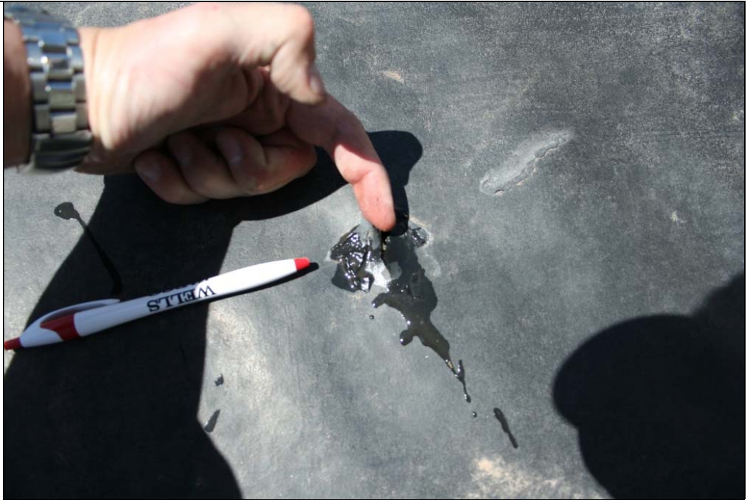
Notes: Detail of hole in Photo 4.
