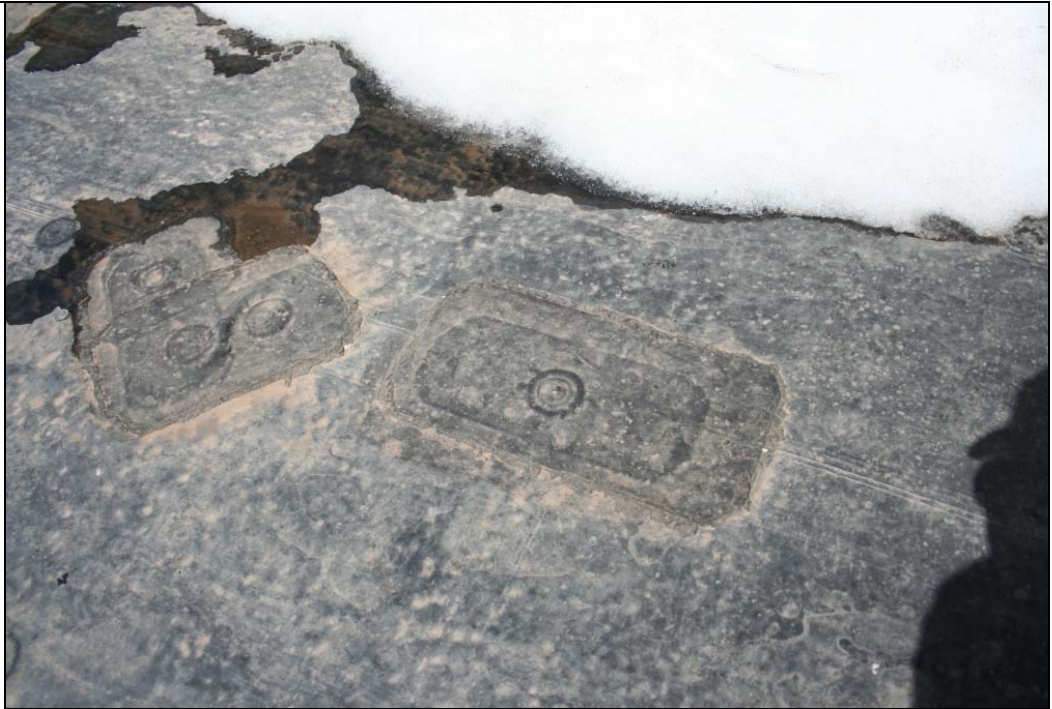
Notes: Patch located southeast of drain.
