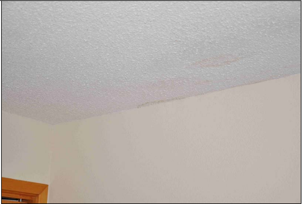
Notes: CBL Interior Photo of drywall damage.
