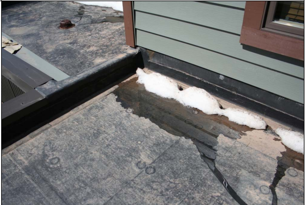
Notes: Ponding water visible in northeast corner.
