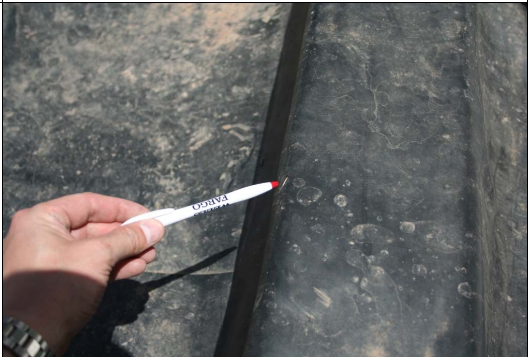
Notes: Gash at south parapet cap.
