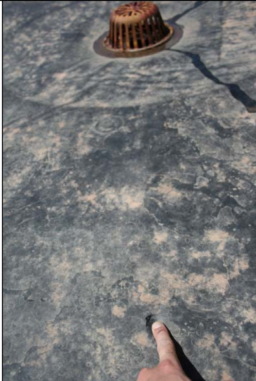
Notes: Location photo of hole 3' south of drain.
