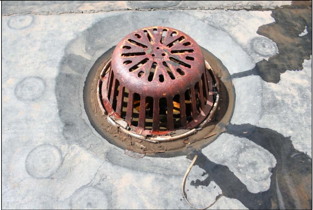
Notes: Debris around perimeter of roof drain.
