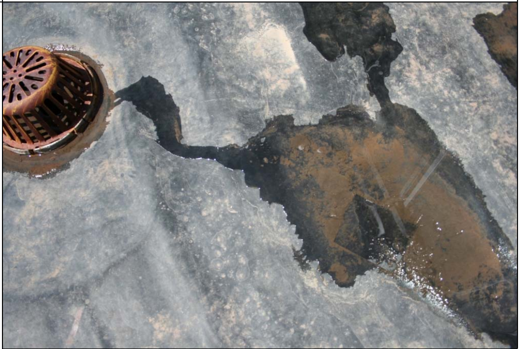
Notes: 1 Patch southeast of roof drain.
