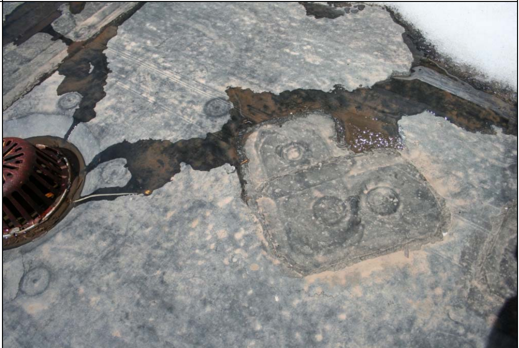
Notes: Patch located southeast of drain.
