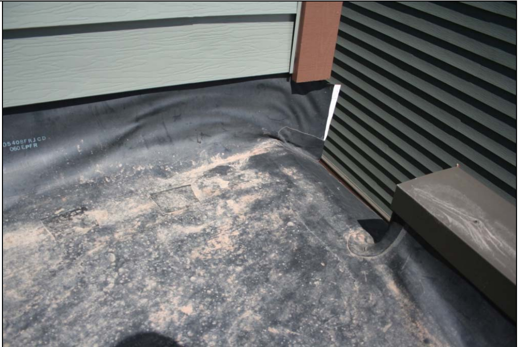
Notes: Detail of overflow scupper and two patches.
