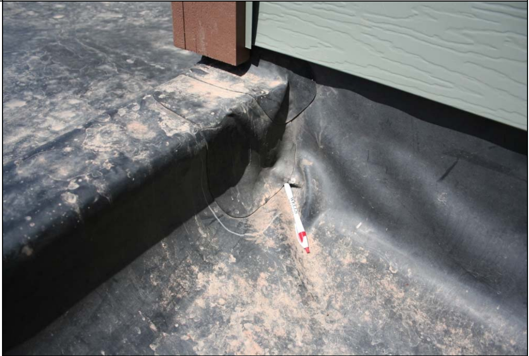
Notes: Corner seam not fully adhered at northeast corner.
