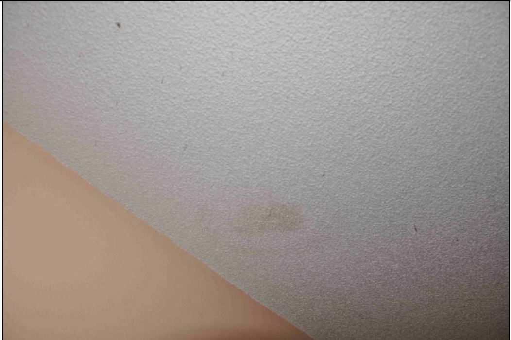
Notes: CBL Interior photo of drywall damage.
